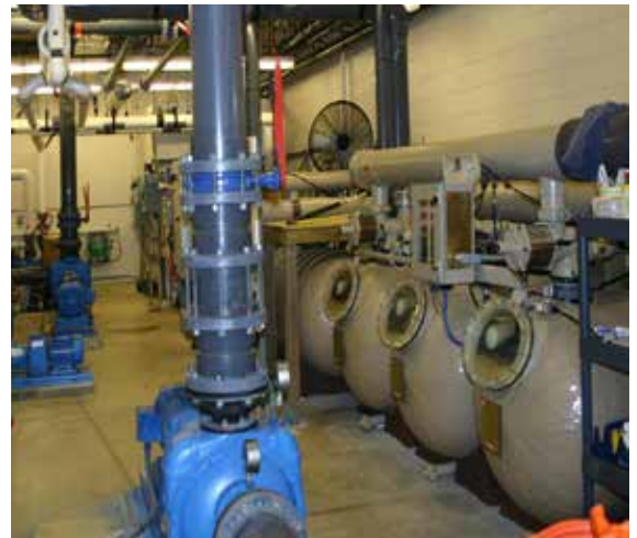
Figure 6-6 Three-Tank Horizontal High-Rate Sand Filtration System
