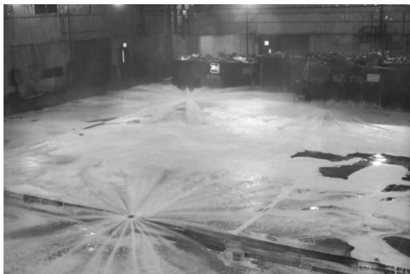
Fig. 4-7 An in-floor sprinkler head in operation
